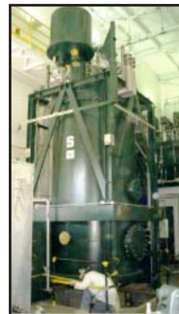
The 1750 watt helium liquifier formerly used by the U.S. Bureau of Mines in Texas and renovated for the NSCL by Jefferson Lab; the 1500 horsepower helium compressor and its backup are in a separate room.
