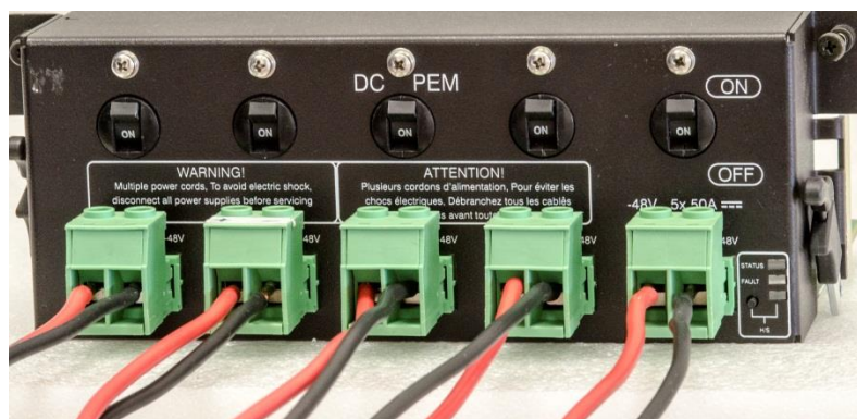
Figure 34: Connection DC Terminal Blocks
