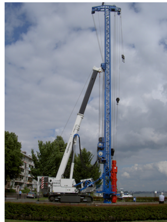
Figure 6.4: Be the first on your block to own a Sennebogen 683 tp telescopic pile driver which can drop 32 tons over a distance of 34.8 meters.
