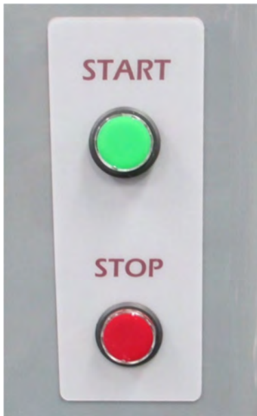
Figure 7-1a: Front Panel of Helium Purification System
