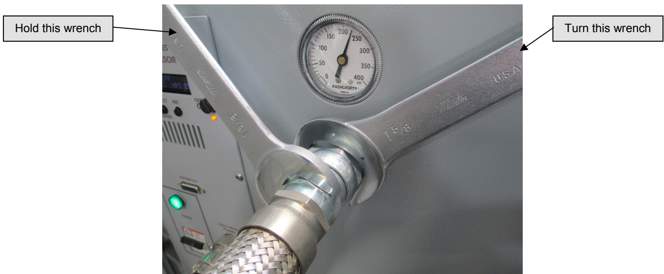
Figure 6-2: Connecting the flex lines to a helium compressor package
