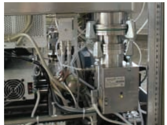
Vacuum Chamber to produce LCD-Displays. Vacuum chamber for filling cholestic liquid crystal materials. Compact Turbo TMH 261, Rotary Vane Pumps Duo 5, Duo 20 and Duo 35, Compact Process Ion Gauge IMR 265 and Valve EVR 116. LC-Tech, Sweden
