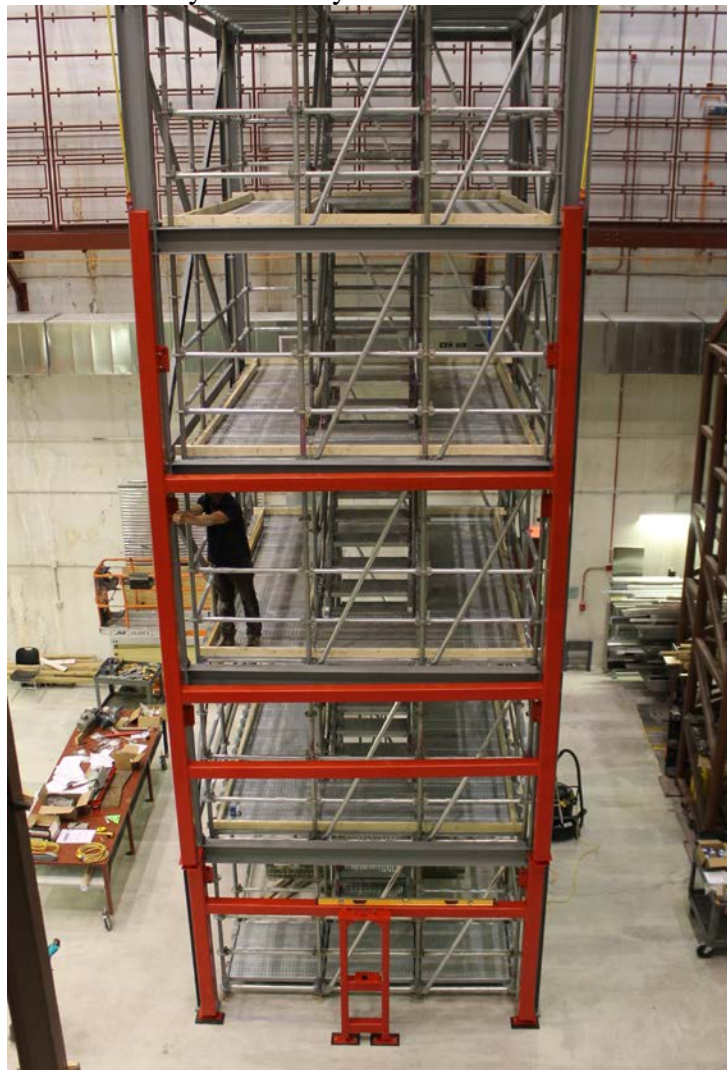
Figure 5: APA Assembly tower with the internal scaffolding in place. The red frame being mounted on the front of the assembly tower is the APA assembly fixture.
